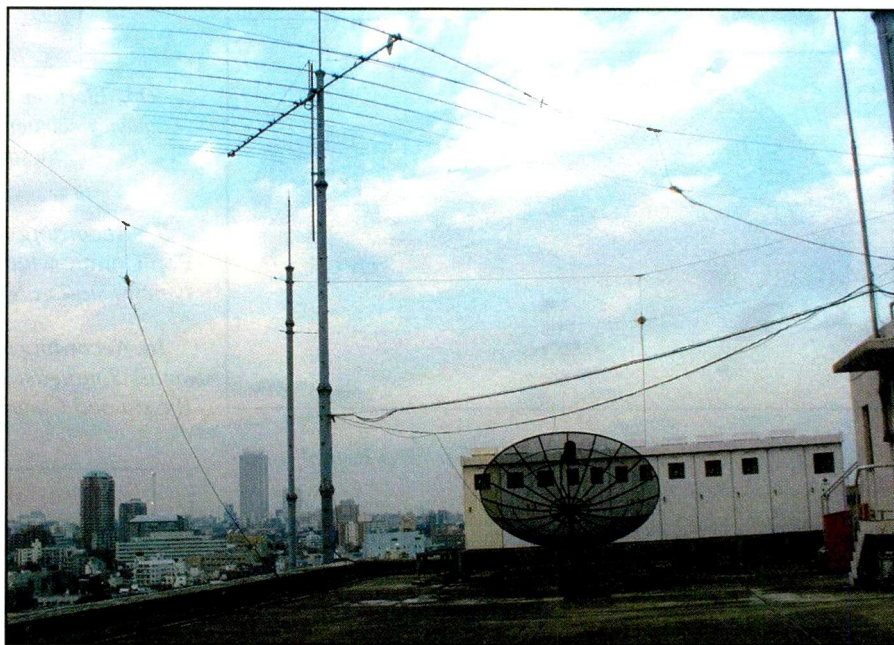
A dish antenna on the rooftop of Radiopress receives TV from a Chinese satellite.
